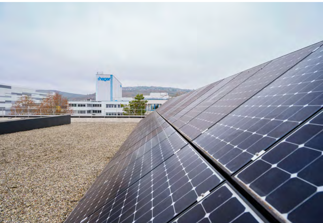
This photo was taken on the roof of Hager Forum in Obernai, France. Hager Forum is first and foremost a meeting place, it also serves as a catalyst for the development of Hager Group. The roof hosts 440 photovoltaic panels that transform solar energy into electric energy. They cover 40% of Hager Forum's energy consumption needs.
